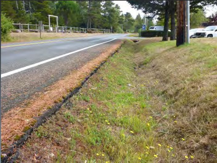
Route 9513 Drainage Ditch & Failing Shoulder #240
