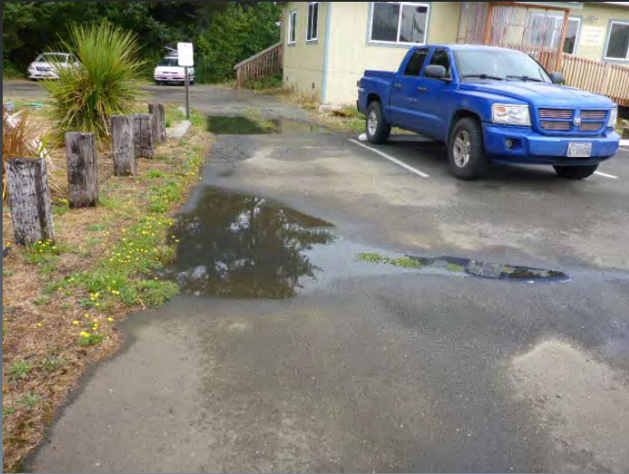
Route 0308 Casino Parking Lot Drainage Issues #125
