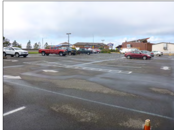
Casino Parking Lot Route 0308 – 11 crashes, 7 involved pedestrians and 4 hit and run. No pedestrian facilities, parking stalls are minimum required and driving lanes are minimum. (Photo #107)
