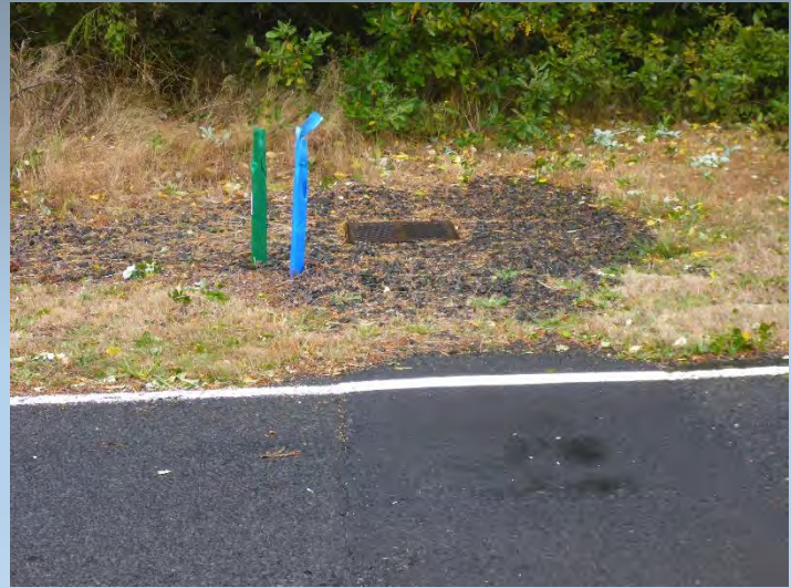
Route 9513 - drainage issues #140
