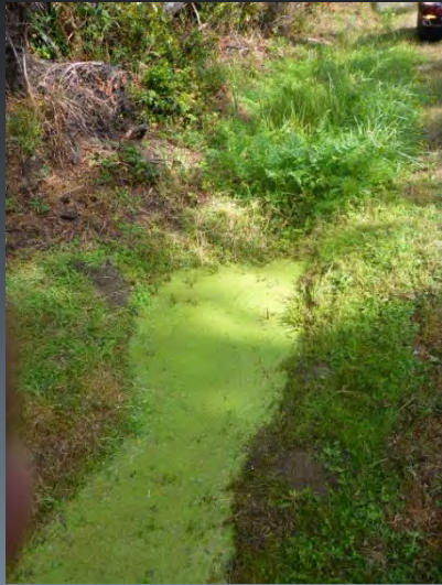
Route 9990 Drainage Issues (Bad Culvert) #265
