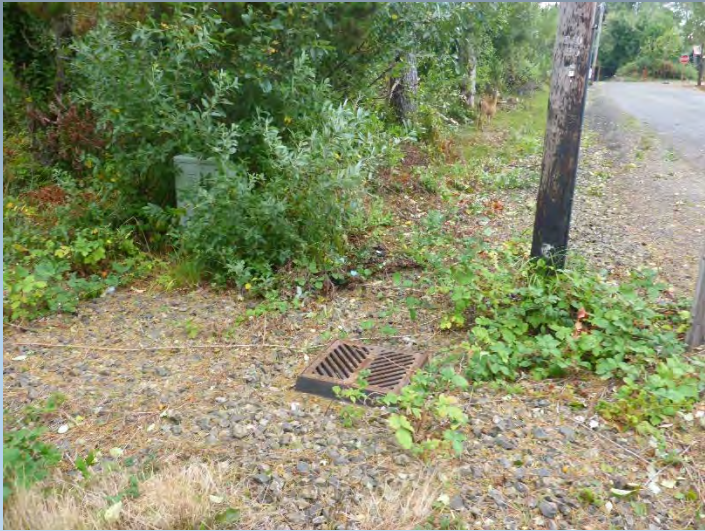
Route 9513 - drainage issues #139
