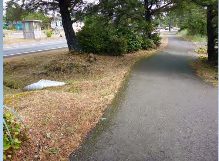
Route 0010 (Asphalt Heaving) #20
