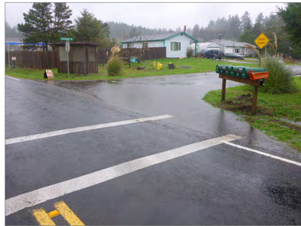
Old Tokeland Rd Route 9513 – Intersection with Shoalwater Bay Dr. Route 0001 – Standing water no drainage, forces pedestrians into roadway. (Photo #164)
