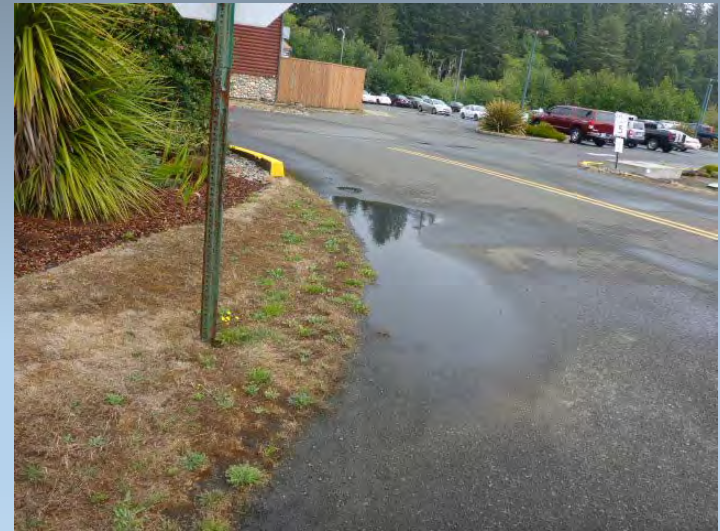
Route 0308 Casino Parking Lot Drainage Issue #124
