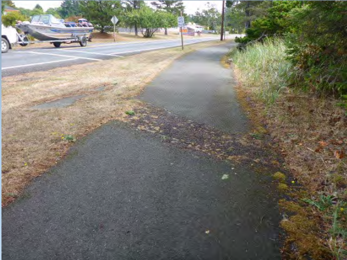
Route 0010 (Bad Longitudinal Patch) #23
