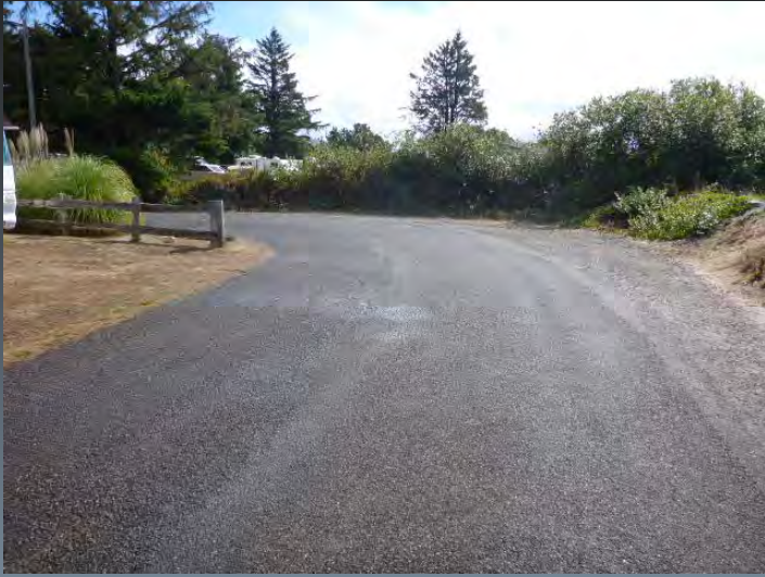
Route 9990 Site Deficiency #273
