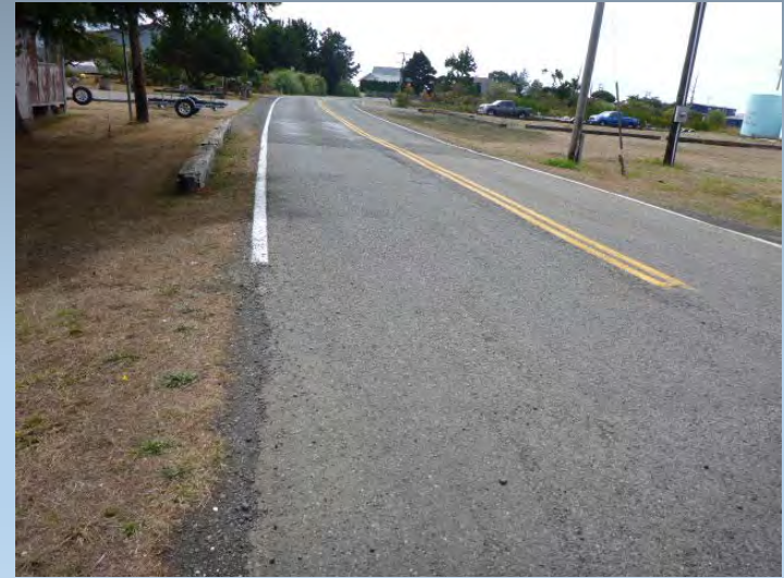
Route 9995 Bad Shoulder #296
