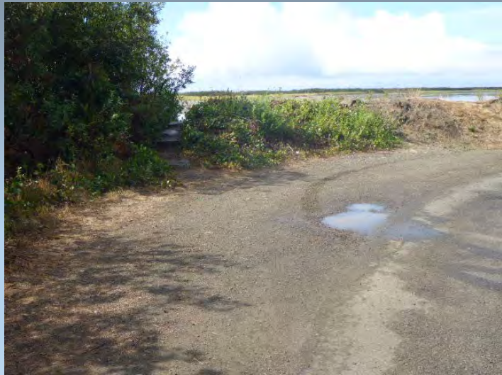
Route 9990 Drainage Issues #267
