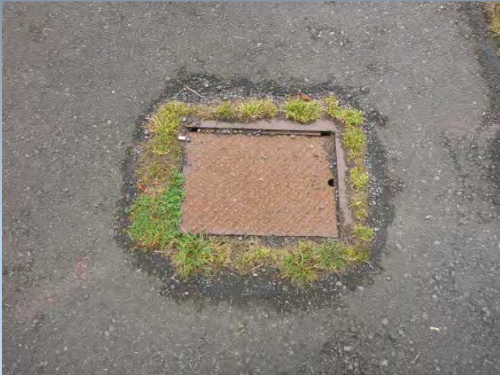
Route 0105 Crosswalk (Trip Hazard) #95
