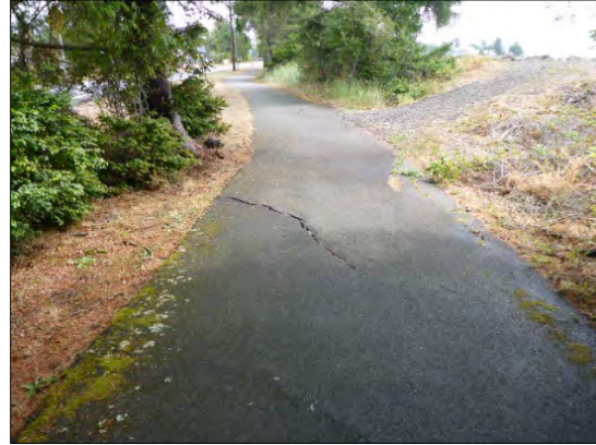
Pedestrian Trail Route 0010 – Pavement heaving, trip hazard. (Photo #21)
