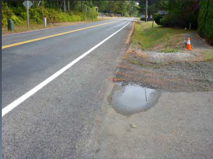
Route 9513 Drainage Issues #252
