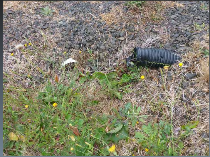
Route 9513 - drainage issues #138
