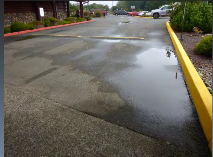
Route 0308 Casino Parking Lot Drainage Issues #126
