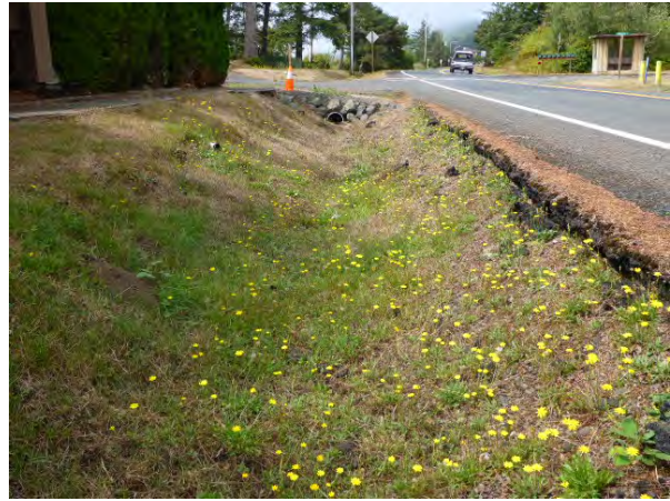
Route 9513 Drainage Ditch & Failing Shoulder (Photo #246)
