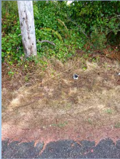
Route 9990 Random Pipe, Possibly for Drainage #271
