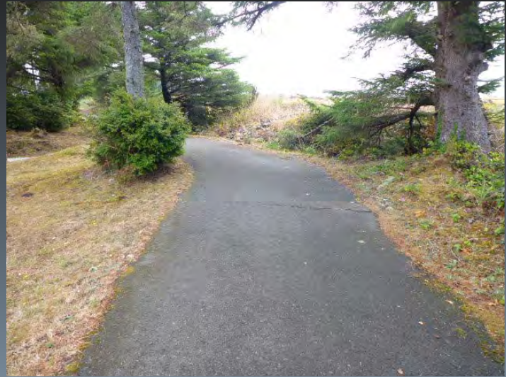
Route 0010 (Asphalt Heaving) #22
