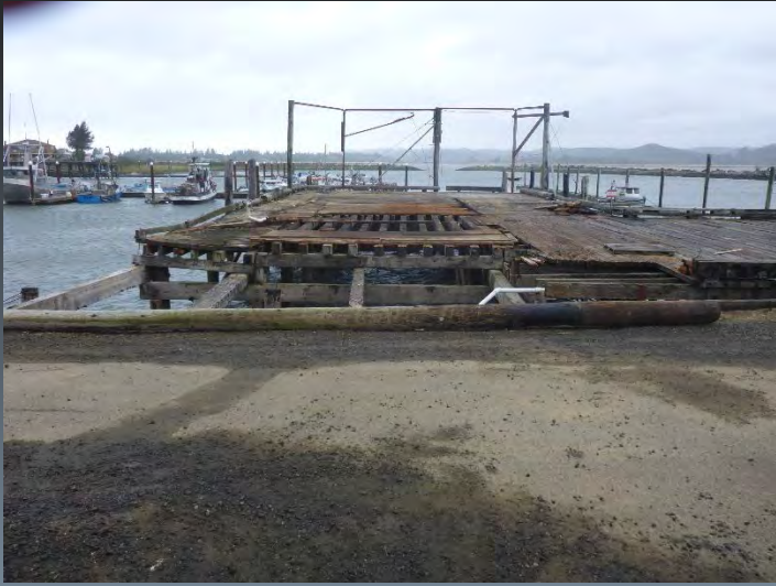
Pier falling apart #5
