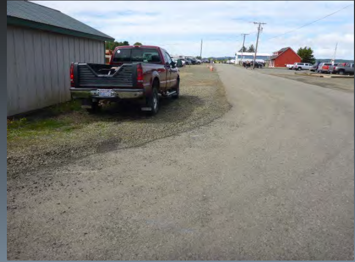
Route 9995 @ Route 0023 Site Dificiencies #286
