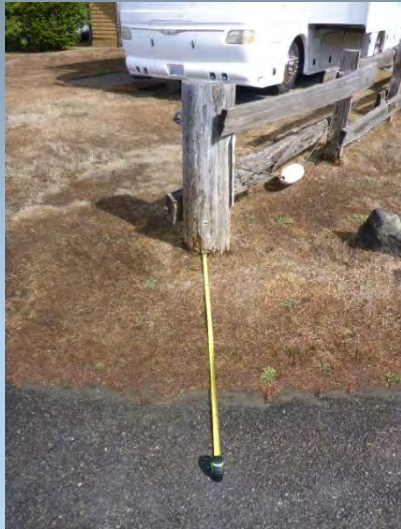
Route 9990 Site Deficiency #275
