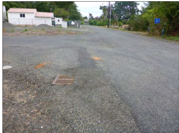
Paul Bunyan Dr. Route 0021 – Intersection with Lagoon Dr. Route 9992 – No stop sign at intersection. No pedestrian facilities. (Photo #52)
