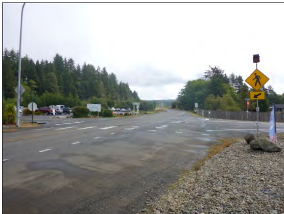
SR 105 Route 0105 – Intersection with Old Tokeland Road Route 9513, Crosswalk faded, crossing signal lights difficult to see in daylight. (Photo #81)
