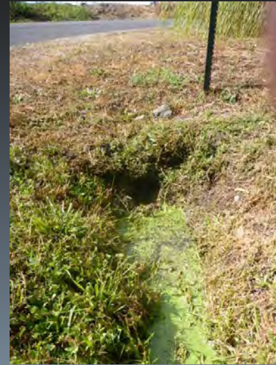
Route 9990 Drainage Issues (Bad Culvert) #266
