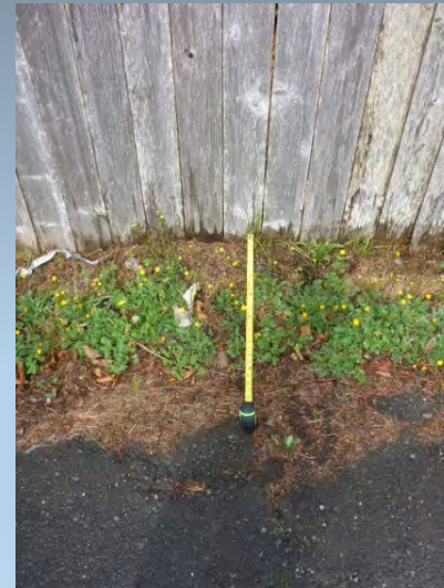
Route 9990 Fence Encroaching Roadway #268
