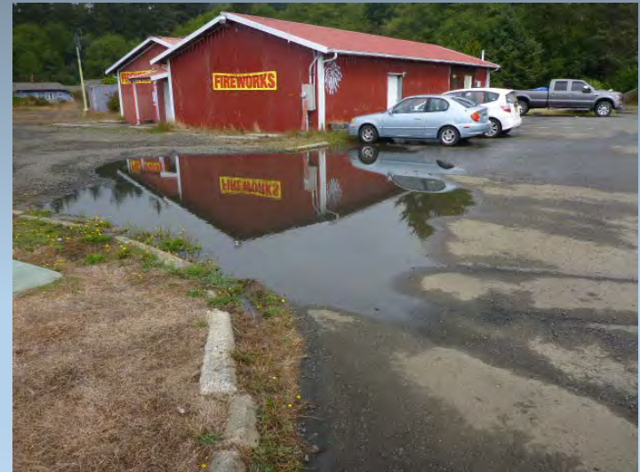
Route 0308 Casino Parking Lot Drainage Issues #128
