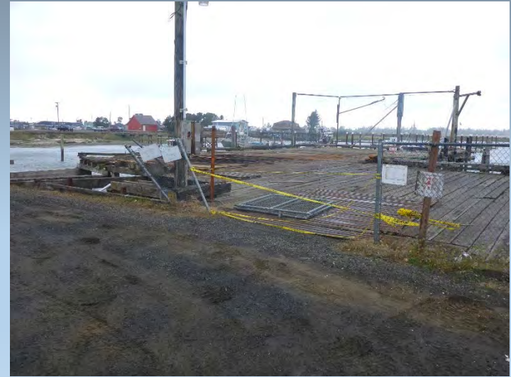
Pier falling apart #4
