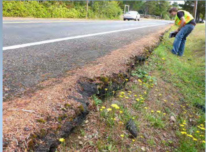
Route 9513 Drainage Ditch & Failing Shoulder #239
