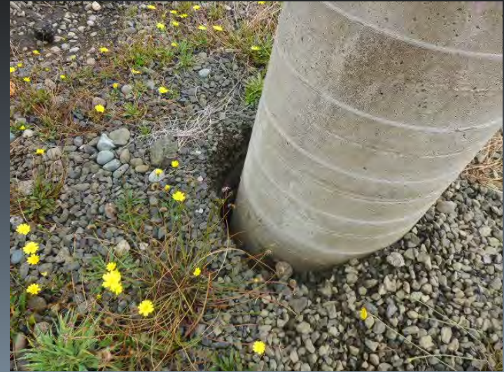
Route 9513 Gas Station Entrance Bad Light Base #253
