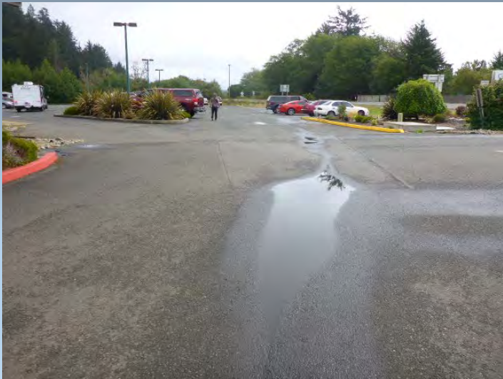
Route 0308 Casino Parking Lot Drainage Issues #127
