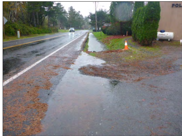
Old Tokeland Rd Route 9513– Intersection and ditch by Police Station. Ditch runs for approximately 1000 feet in length and 2 feet deep. Hazardous to vehicles, the runoff and the edge. (Photo #169A)
