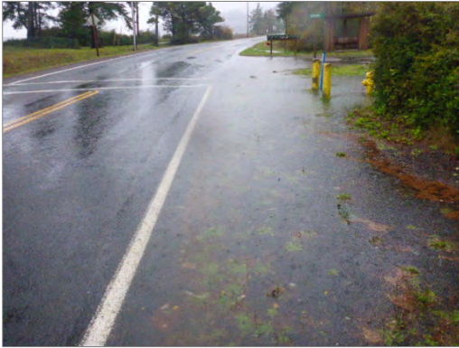
Old Tokeland Rd Route 9513- Northeast side of roadway. Standing water forces pedestrians out into traffic. (Photo #143)
