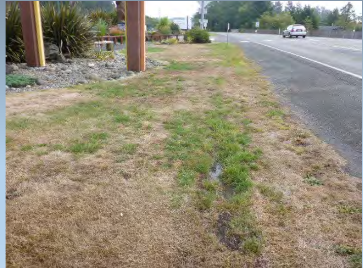
Route 0105 Drainage Issues Shoulder #96
