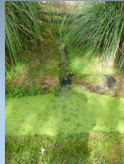
Route 9990 Drainage Issues (Bad Culvert) @264
