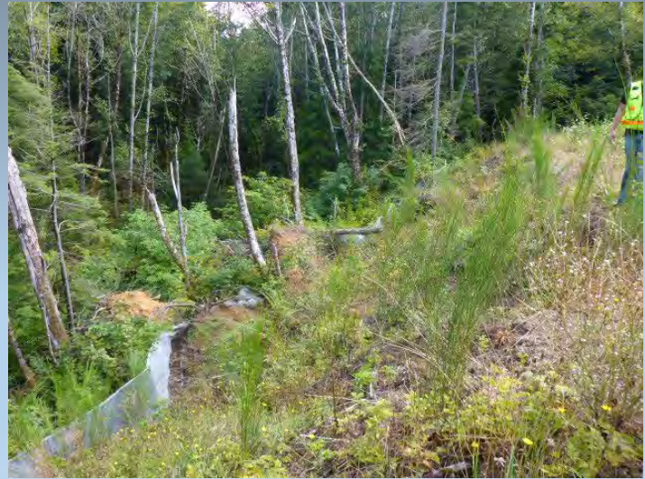
Route 0003 New Building Back Hillslope Failing #12
