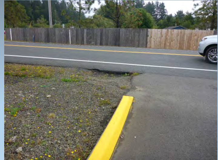
Route 9513 Gas Station Entrance Failing Shoulder #255
