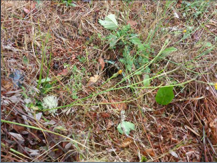
Route 9513 - drainage issues #141
