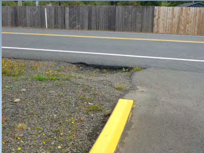
Route 9513 Gas Station Entrance Failing Shoulder #254
