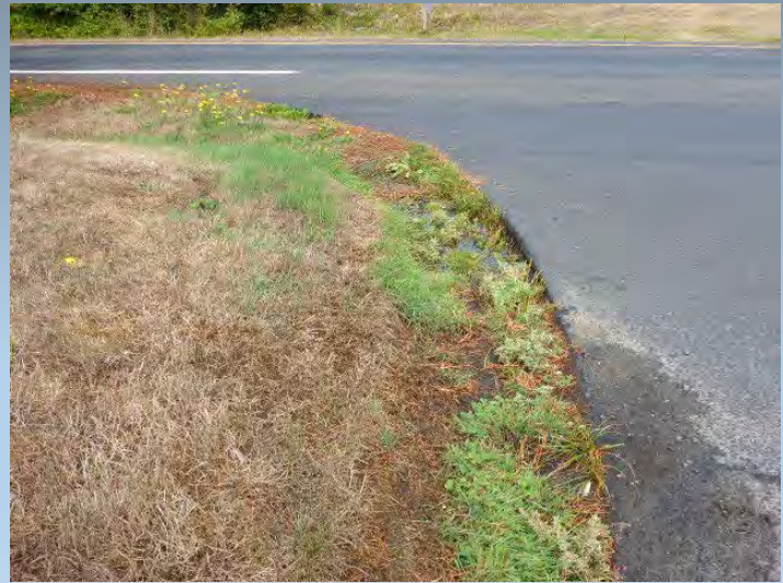
Route 9513 Drainage Issues #251
