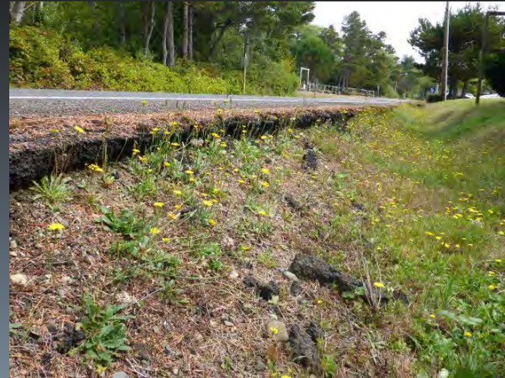
Route 9513 Drainage Ditch & Failing Shoulder #241
