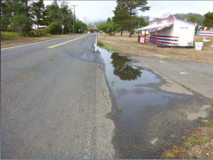
Route 9513 @ Route 9994 (Drainage Issues) #216
