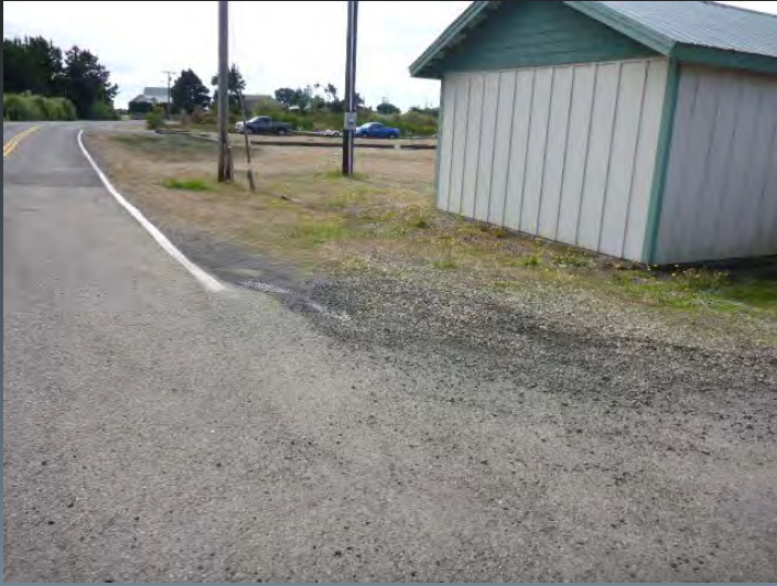
Route 9995 @ Route 0023 Site Dificiencies #285
