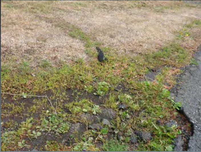
Route 9513 Bad Road Shoulder & Buried Culvert #236
