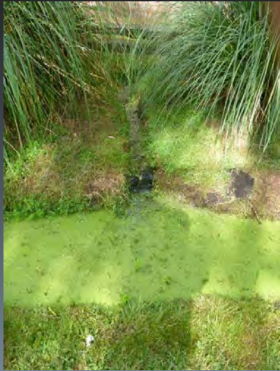
Route 0028 Drainage Issues #77
