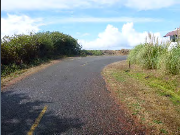
Route 9990 Site Deficiency #277
