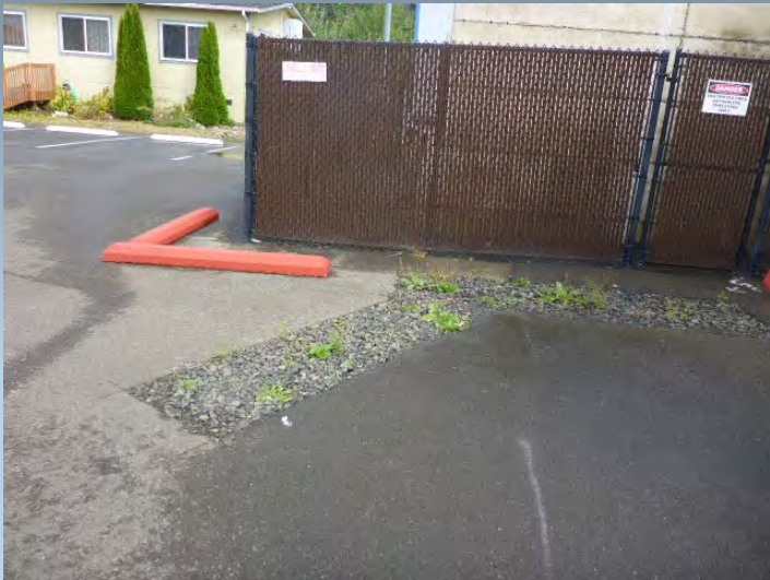
Route 0308 Casino Parking Lot (Saw Cut Not Patched) #123
