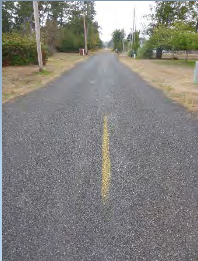
Route 9990 - worn striping #263
