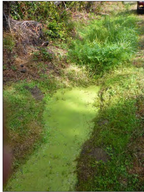
7 th St. Route 0028 – Plugged drain pipe with no place to drain. (Photo #78)
