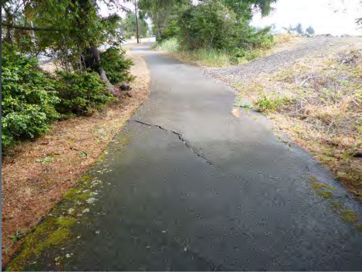
Route 0010 (Asphalt Heaving) #21
