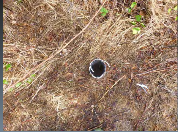
Route 9990 Random Pipe, Possibly for Drainage #270
