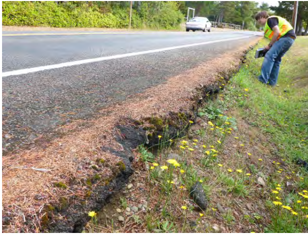
Route 9513 Drainage Ditch & Failing Shoulder (Photo #239)
